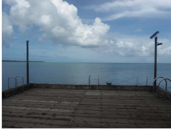
Figure 3. Merizo pier with missing solar lights.
